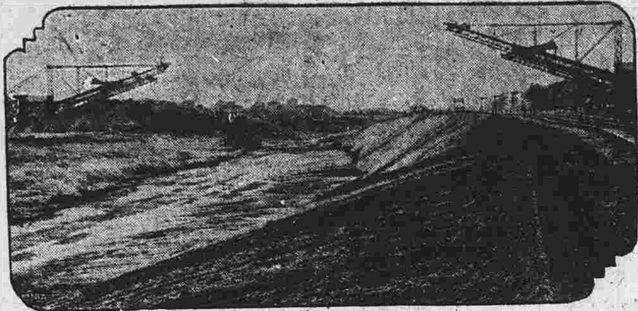
Here is a comprehensive view of a section of the River Shannon Power Canal at the Black Water end. Near here is to be located the dam which indirectly will provide the 90,000 electrical horsepower.
